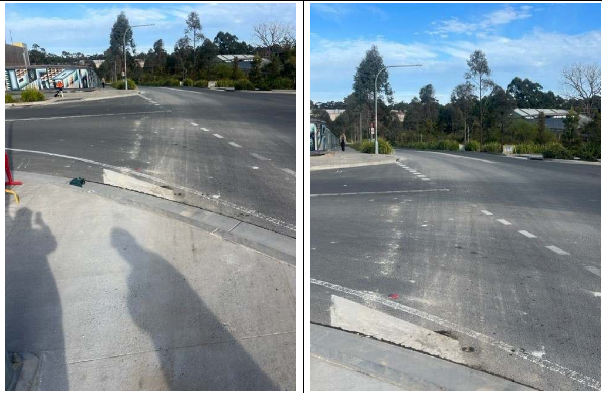
Photos 17 & 18: Minor tracking was observed from the work zone / VENM load-out zone onto De Clambe Drive
