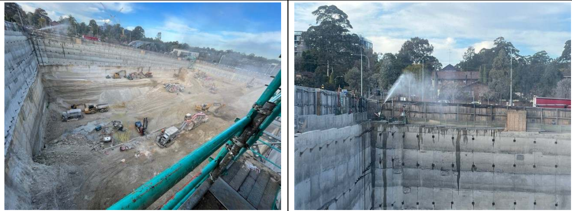
Photos 19 & 20: Excavation of the basement structure was ongoing. Water cannons were in place to reduce dust
